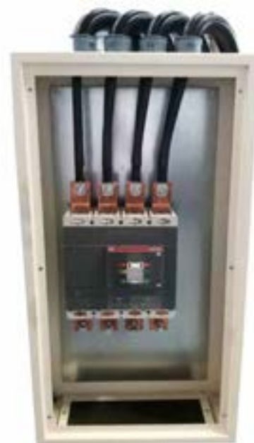
Protection Switch Panel
